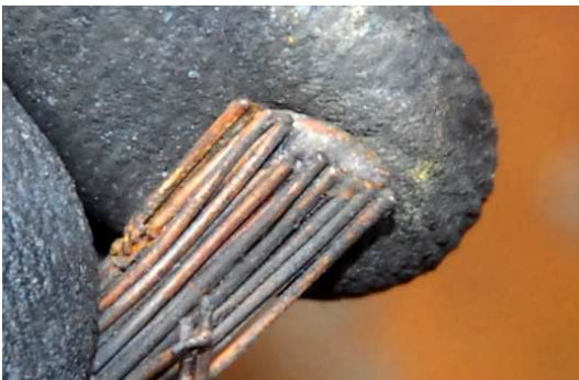
Figure 5: Example of arc bead on a supply conductor to a starter motor.
