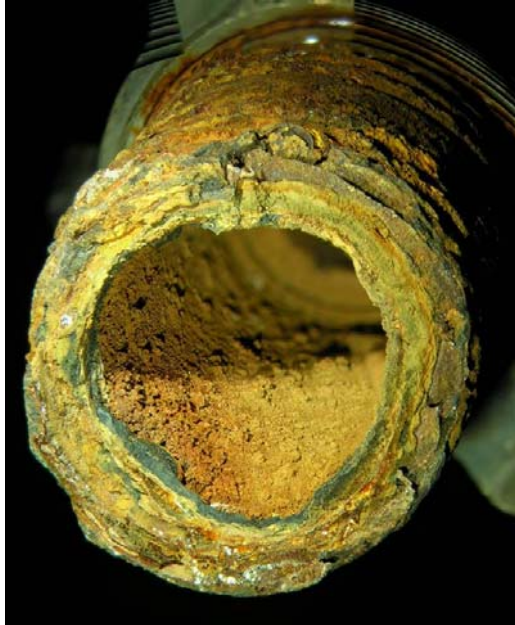
Galvanic corrosion failure of a steel pipe nipple interconnecting two stainless steel fittings
