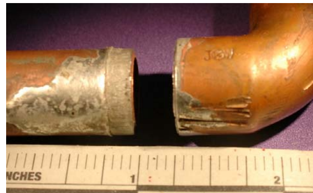
Separation of soldered pipe joint due to insufficient insertion into cup
